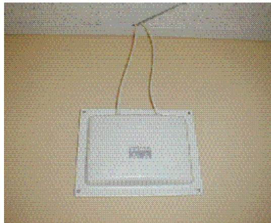
Figure 13. Figure 9 Cisco Aironet 2012 Antenna Mounted to a Wall
