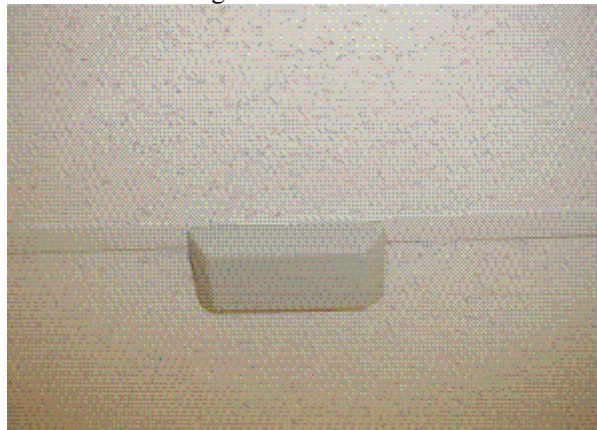
Figure 11. Cisco Aironet 5959 Antenna Mounted to a Ceiling
