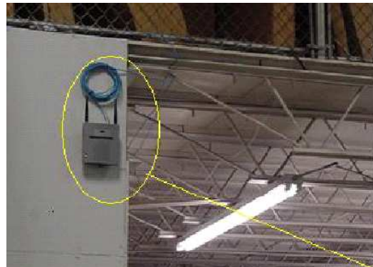
Figure 8. AP and Antennas Mounted on a Wall, Away from I-Beams
