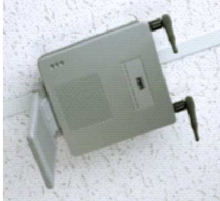
Figure 10. Cisco AP1200 Mounted to a Ceiling
